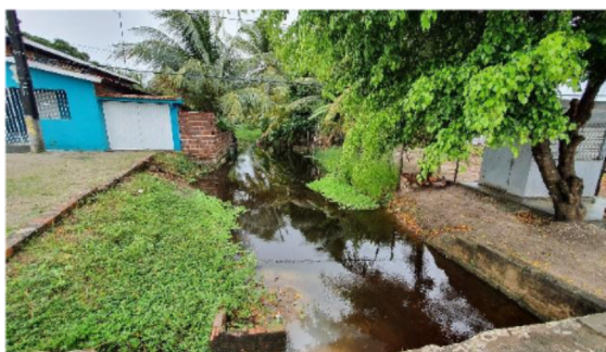
P3. Vala esgotamento (S07°32'16,3" W034°49'43,3")
